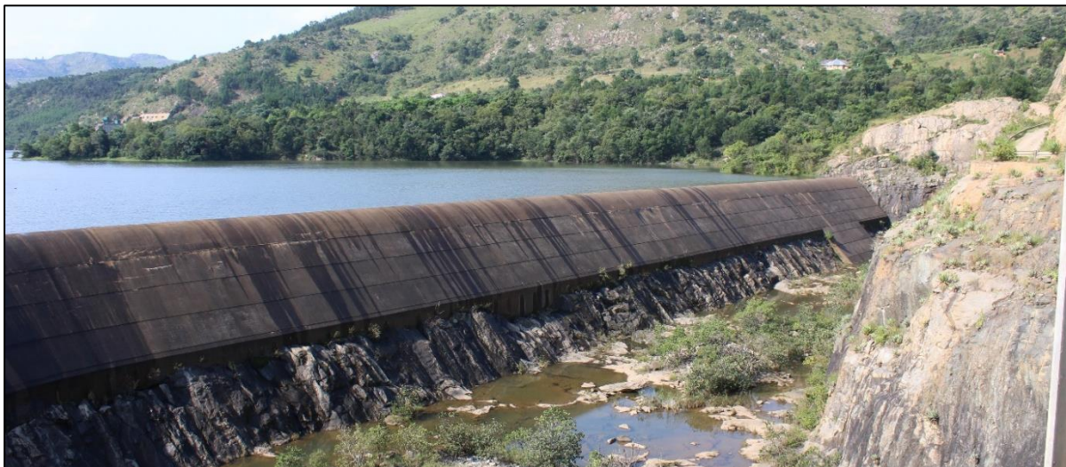
Figure 7-13: The Luphohlo Dam on the Lusushwana River Upstream of the Proposed Nondvo Dam
