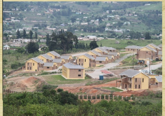
Construction of Institutional housing at the TB Centre in Manzini which is in it's final stage
