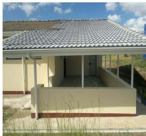
Figure 2: Renovations at Dvokolwako TB/HIV clinic including reconstruction of the patient waiting area supported by URC in the Hhohho region
