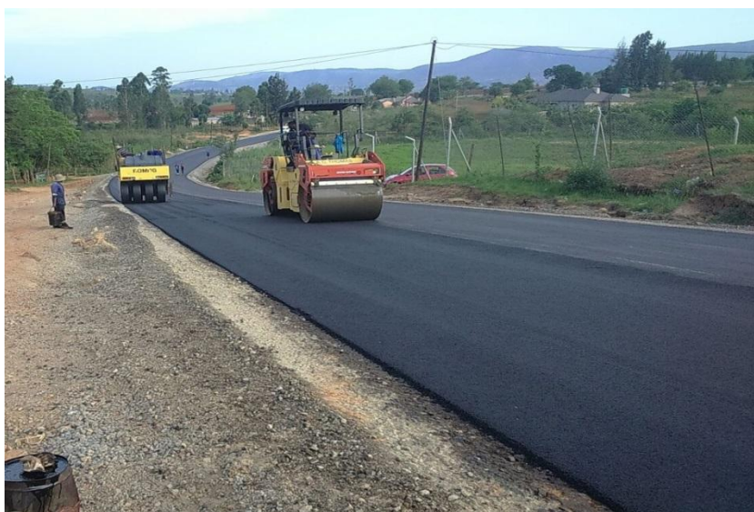
Resealing of Njingeni—Malkerns Research Station Road & access road to Vulamasango Correctional Facility
