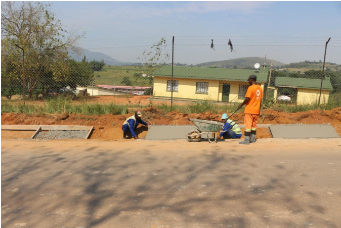
On-going works (construction of drainage systems) at Njingeni – Malkerns Research Station road
